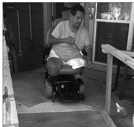
Nina Lozano can enter and exit her apartment safely, thanks to repairs made by volunteers from the Austin Chapter of the Texas Ramp Project.
